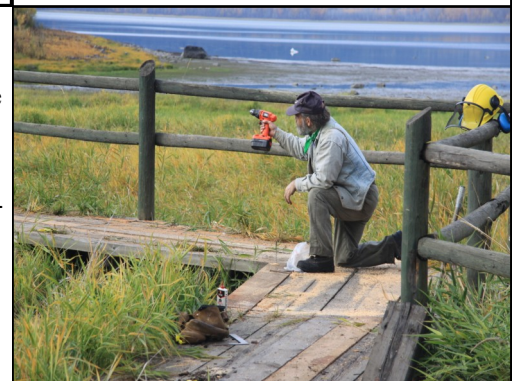
John repairing one of the boardwalks He loved to be out on the trail
